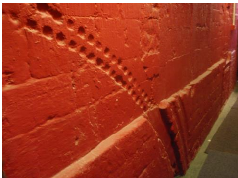
Arc where barring plate was mounted
